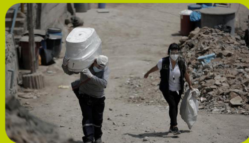
Installation of off-grid, urine diverting toilet
